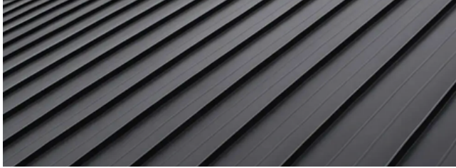
METAL ROOF ACCENTS
