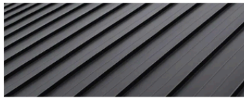
METAL ROOF ACCENTS
